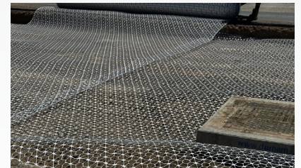
Rolling out the Tensar InterAx geogrid on the Lawrence Street pavement site.
